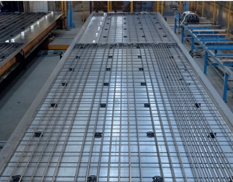
The spacers are placed accurately and a steady rate of concrete coverage is thus guaranteed. The savings potential is considerable.
